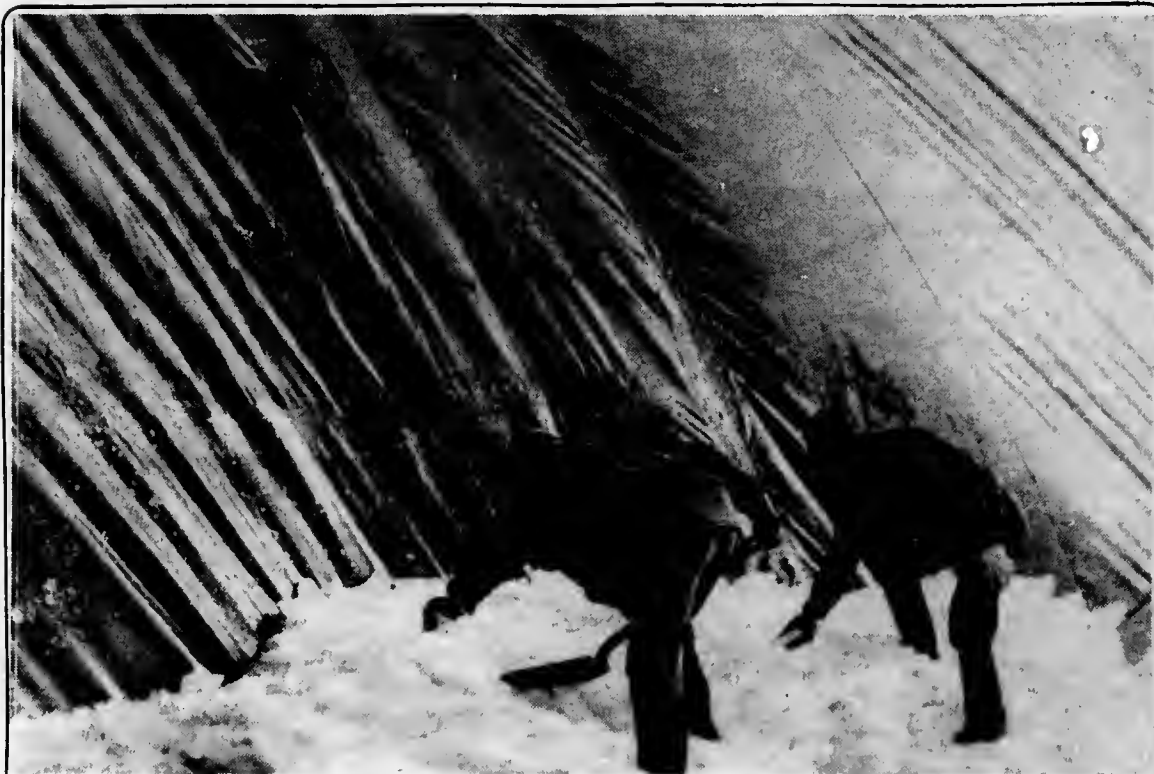
Bubble trouble — Workers shovel icy rubble to repair Bubble after snow piled on top
