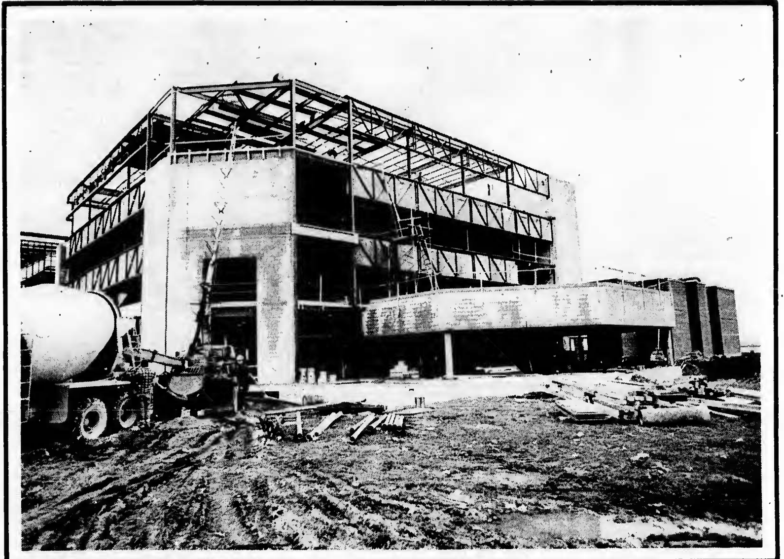
Construction continues on Phase 3. Workers are fighting a continuing battle against the encroaching tentacles of Old Man Winter. Expected completion date is in 1973.
