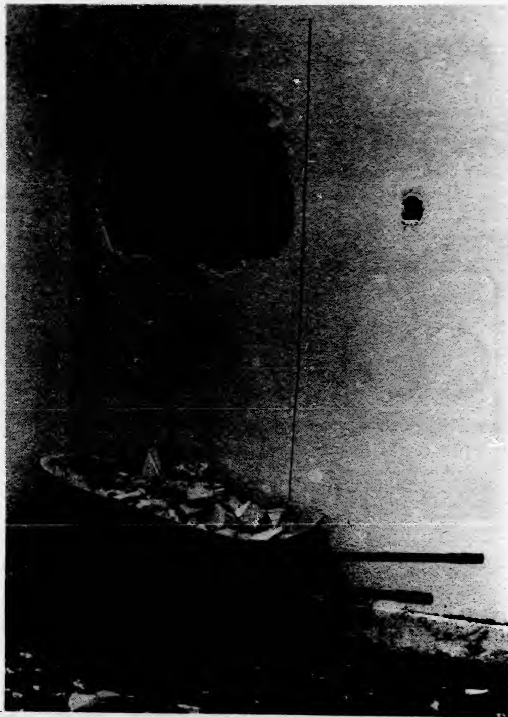
Daycare — A maintenance man knocks a hole in the wall near Continuous Learning to make room for a door into the Daycare Centre. The Centre opens today.
