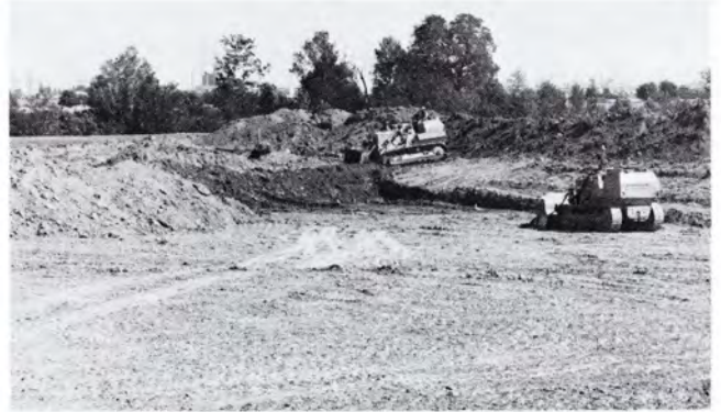
Construction workers clear the ground for new parking lot at Humber's North Campus.
