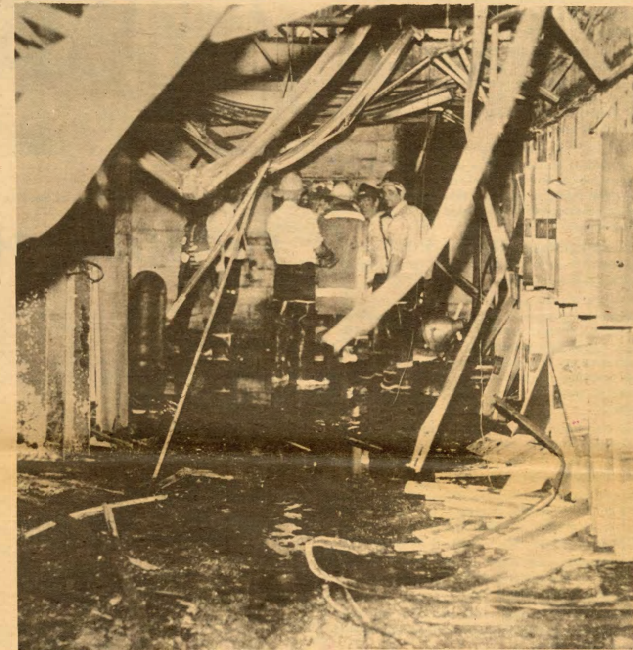
Fire investigators were confused by the amount of fire damage in the fieldhouse. The fieldhouse was supposed to be a low fire risk area.
