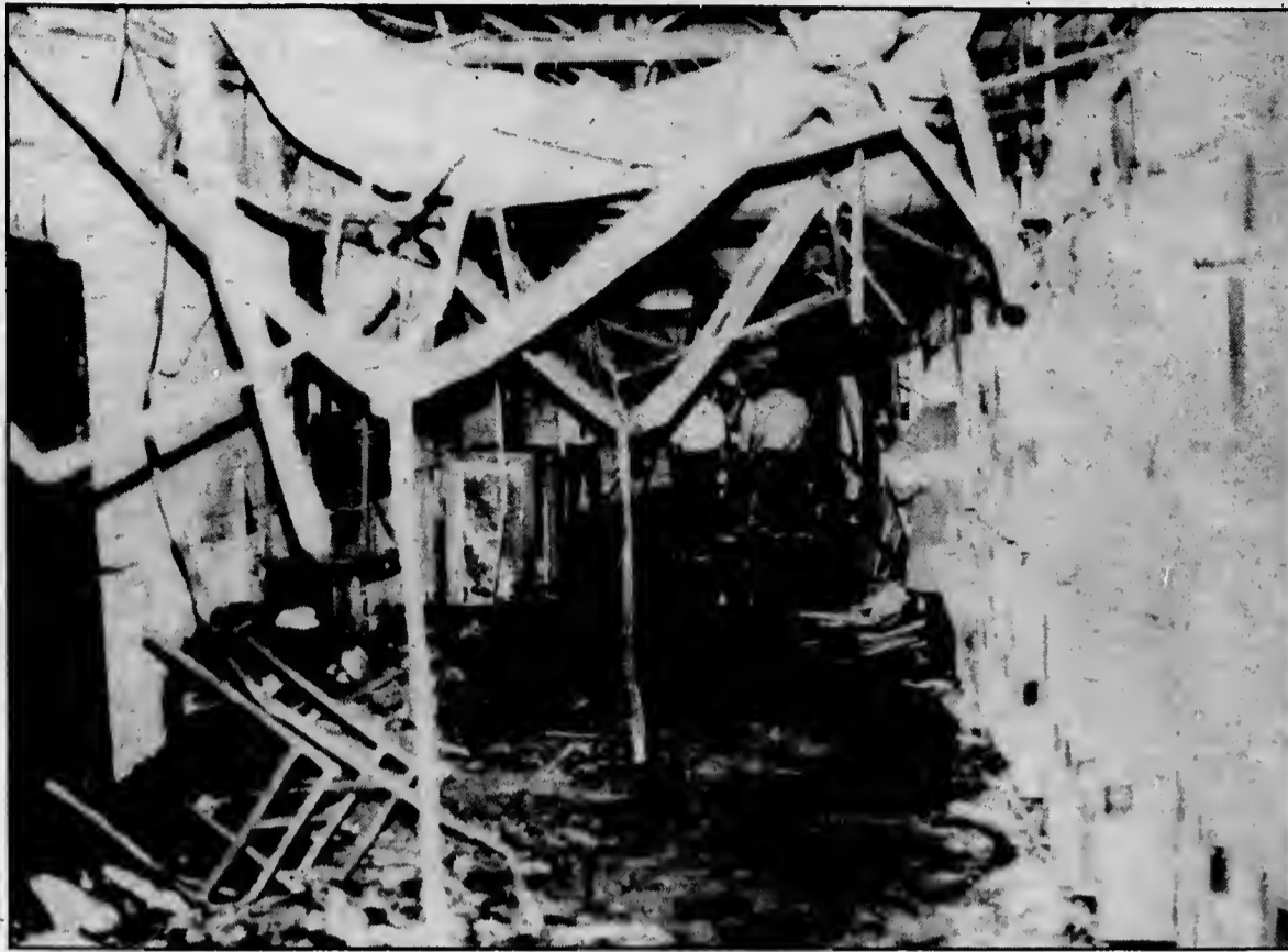
THE DAMAGE —This fire in D-block was one of seven fires in 1973 caused by arson. Damage in this fire was estimated at $1,250,000.
