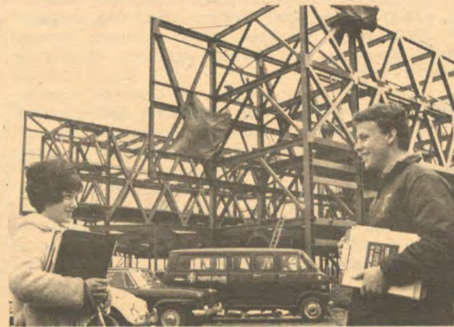
Phase II of Humber's building program is well underway, and will eventually be the permanent home of Business Division. Here Ruth Fisher and Rick McGee discuss the new steel superstructure. The addition is scheduled for occupancy in October.
