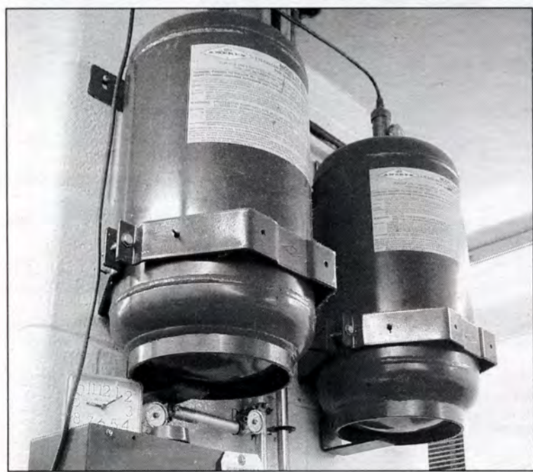
Fire suppression equipment disperses a chemical designed to put out fires on stoves and other cooking areas at Humber.
