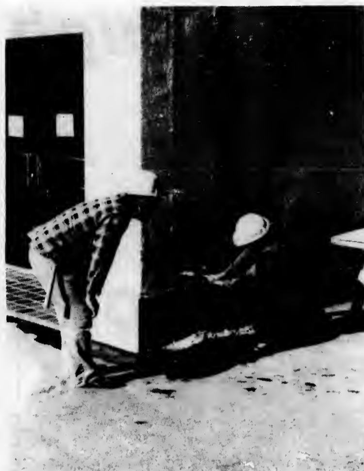
Workers prepare wall outside "E" Building to confirm measurements needed to begin construction.
