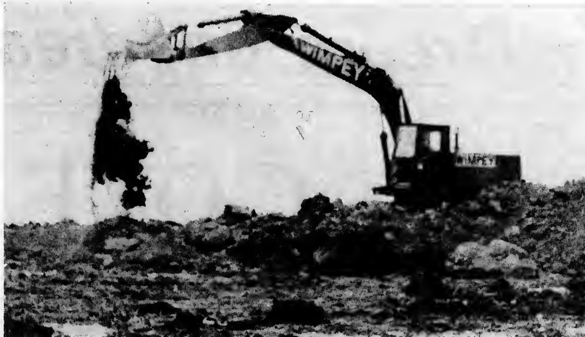
Diggin' for gold —Construction of new homes begin near North Campus after Etobicoke froze development ten years ago.
