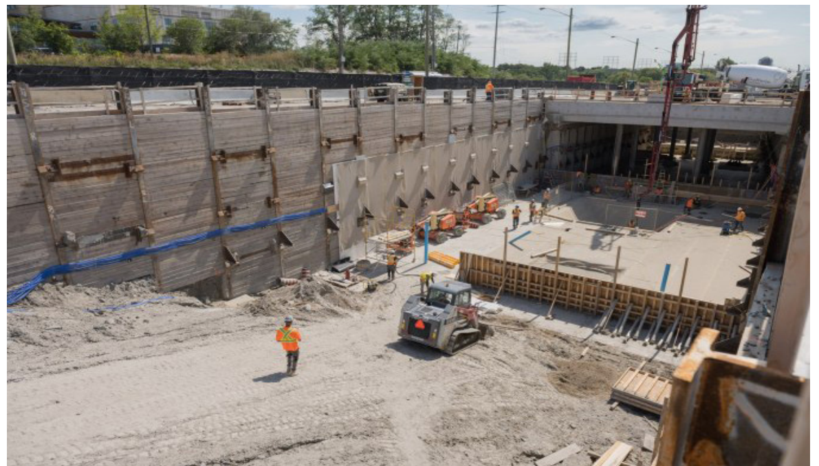
This is where the Light Rail Vehicle (LRV) will enter and exit the station at Humber College. Concrete pours are continuing for the station's base and preliminary construction for track installation starts later this year.
